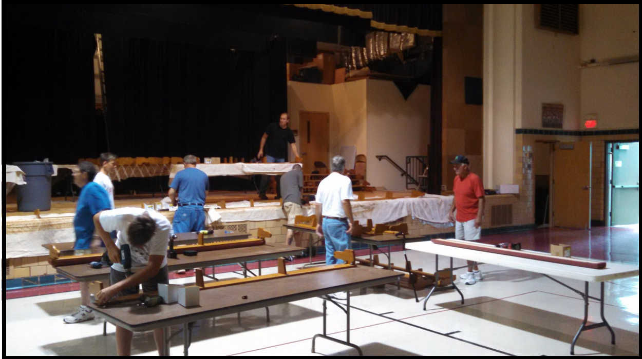
The kneelers removed from the pew and worked on in the School Gym.
